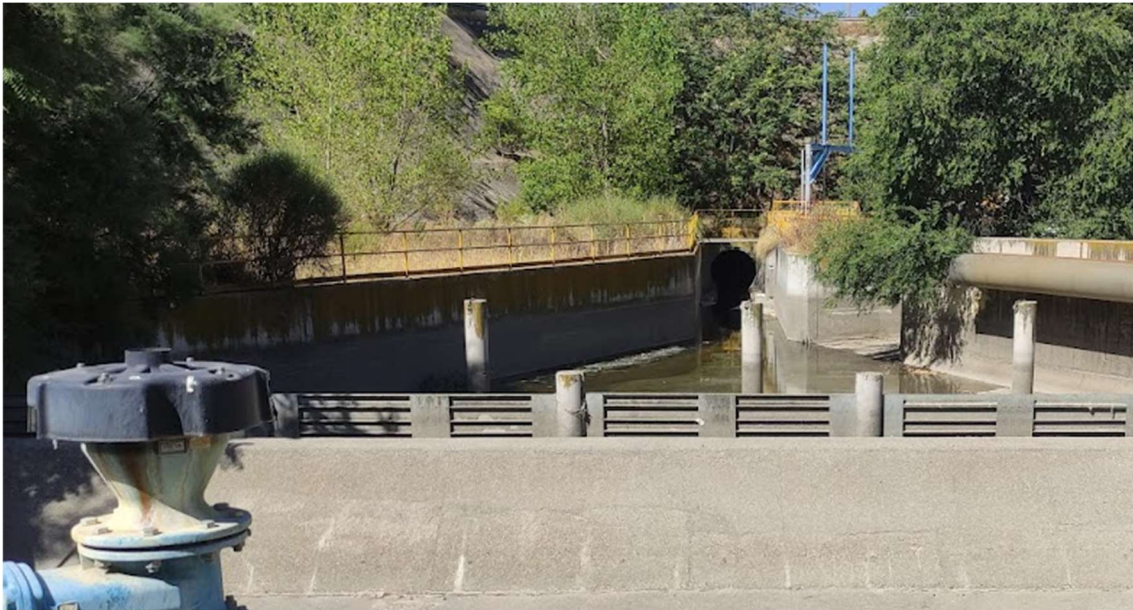
Figure 5. Butarque II collector reaching the CSO chamber, where it can be observed that it is a very deep collector
