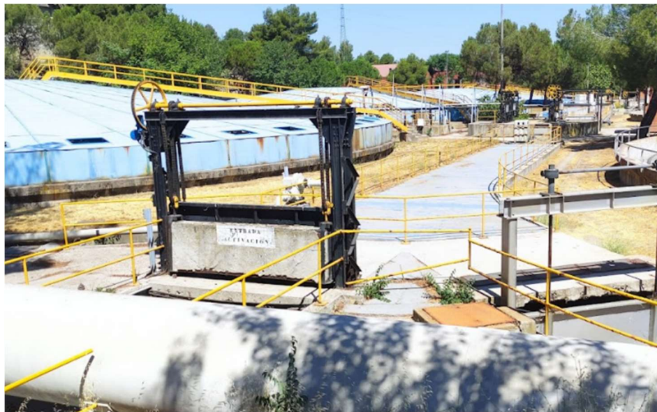
Figure 15. Water channel driving the waters from the primary to the secondary treatment. At the left waters are driven to the secondary while whenever the biological capacity is surpassed the waters are driven right to the river.
