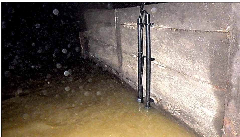
Sensors installed in the sewer:
