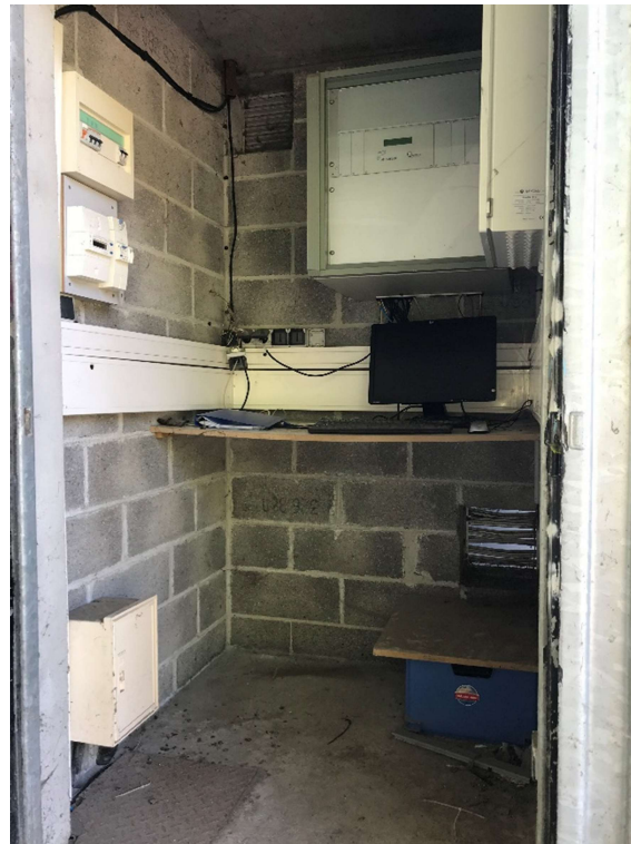
Figure 5 : Internal view of the D3 station (Marina of Wembrechies).
