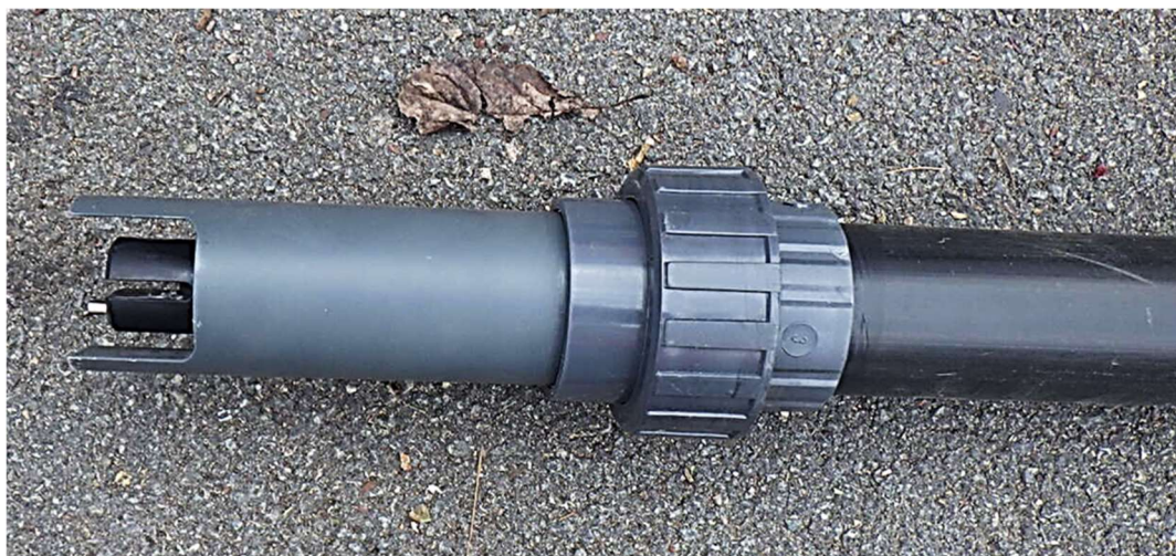
Conductivity sensor fixed on the PVC protective pipe
