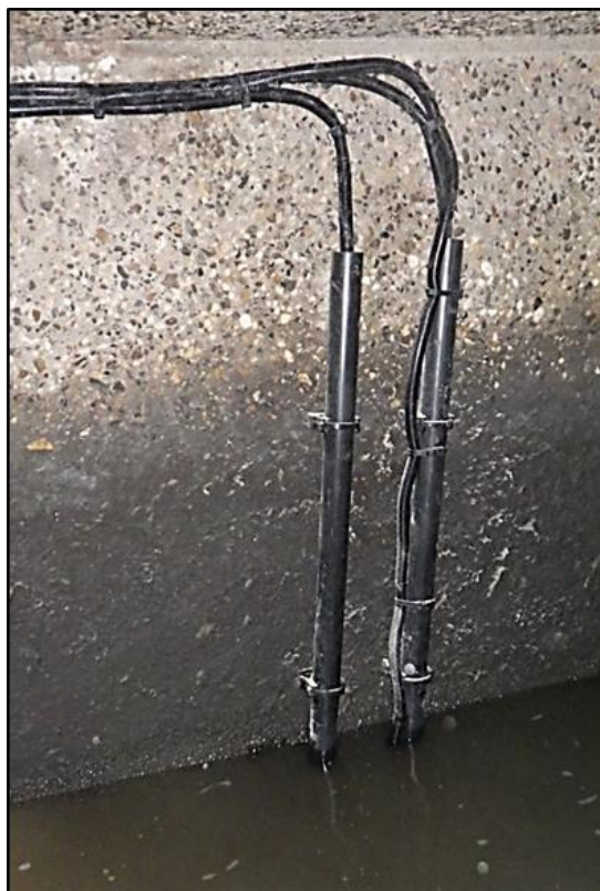
Figure 14 Sensors installed in the sewer of PC527-101 Sainte Hélène Thiers
