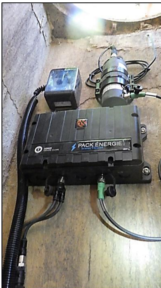
Figure 17 Data logger, battery pack and programmer for the turbidity probe cleaning system of Weir 350-001 Bâteliers
