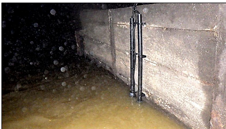
Figure 18 Sensors installed in the sewer of Weir 350-001 Bâteliers
