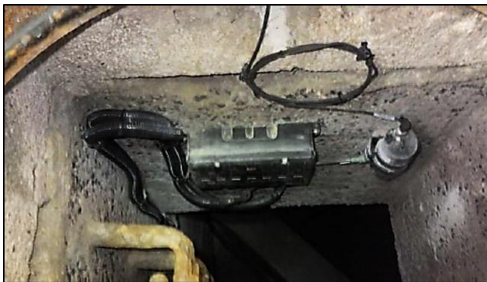
Figure 10 Data logger and battery pack of Weir 328-001 Café des fleurs
