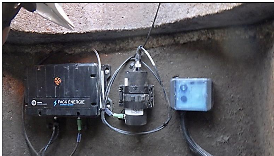
Figure 15 Data logger, battery pack and programmer for the turbidity probe cleaning system of PC527-101 Sainte Hélène Pasteur
