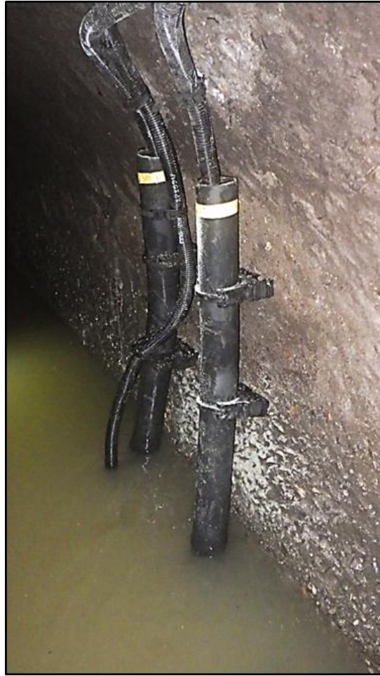
Figure 16 Sensors installed in the sewer of PC527-101 Sainte Hélène Pasteur
