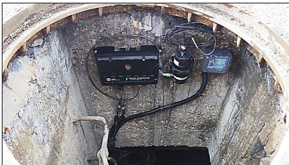
Figure 13 Data logger, battery pack and programmer for the turbidity probe cleaning system of PC527-101 Sainte Hélène Thiers
