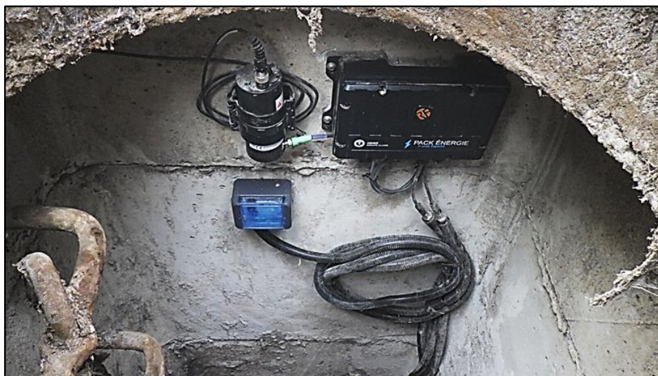
Figure 19 Data logger, battery pack and programmer for the turbidity probe cleaning system of weir 350-002 Maracci
