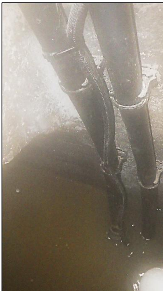
Figure 20 Sensors installed in the sewer of weir 350-002 Maracci
